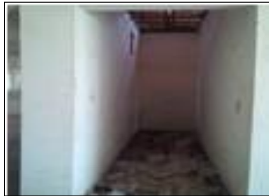
Fig 1: The Removed Ceiling Tiles (Source: Authors' Field Work, 2018).
