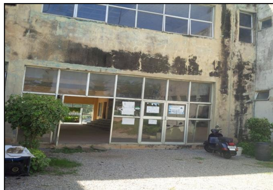
Fig 2: Faded and Peeling Wall Paint (Source: Authors' Field Work, 2018).
